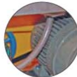
Pump is gravity-fed from tank.
